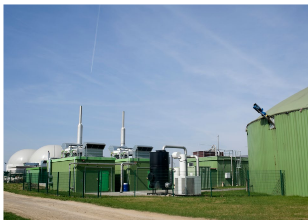
Two generators using biogas, and digesters
