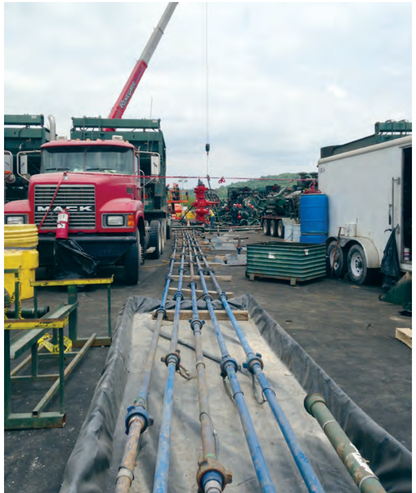
Completion equipment at a gas well.
