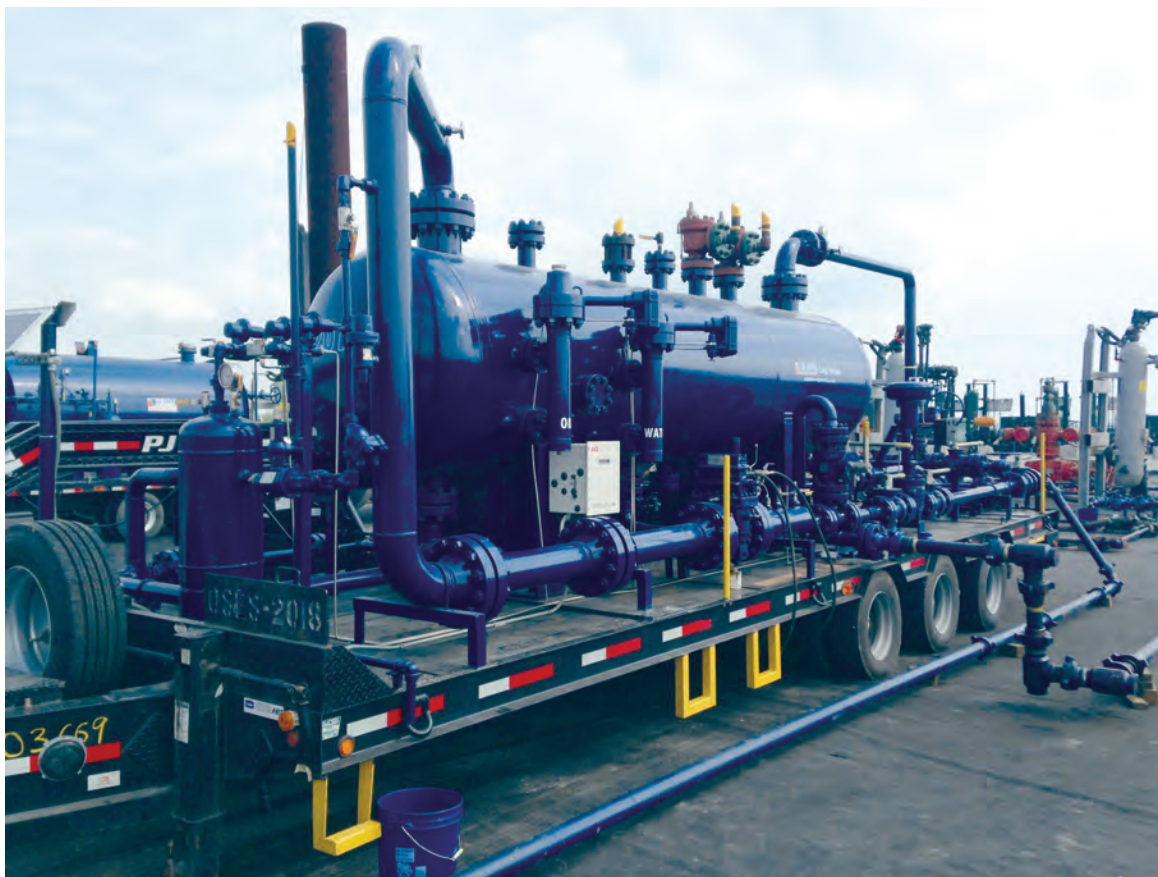
Equipment at a gas well.
