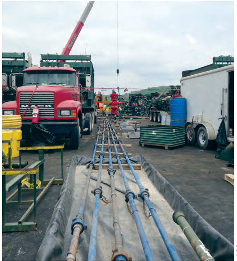
Completion equipment at a gas well.
